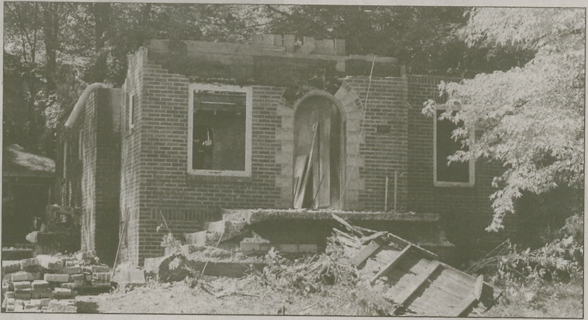
Deconstruction of this house at 945 Brentwood Ave. will cost $4,400, but will keep brick, stone and lumber out of the landfill.
